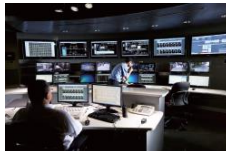
Command and control center
